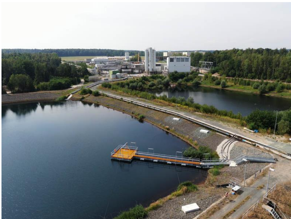
Figure 4-25. Water treatment plant WTP in Königstein with settling bassins prior to water discharge to the Elbe river
